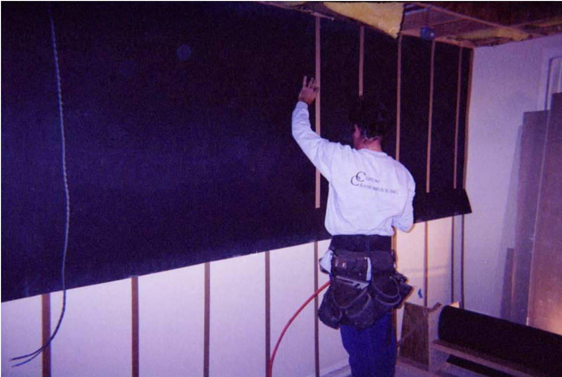
Photo 1 – First layer of shims and first course of Acoustiblok and top shim installation. (Note the roll dispenser in the background made from scrap 2x4, \frac{3}{4} plywood, and a length of galvanized pipe. The pipe rests in V notches in the plywood uprights, making it easy to load new rolls.)
