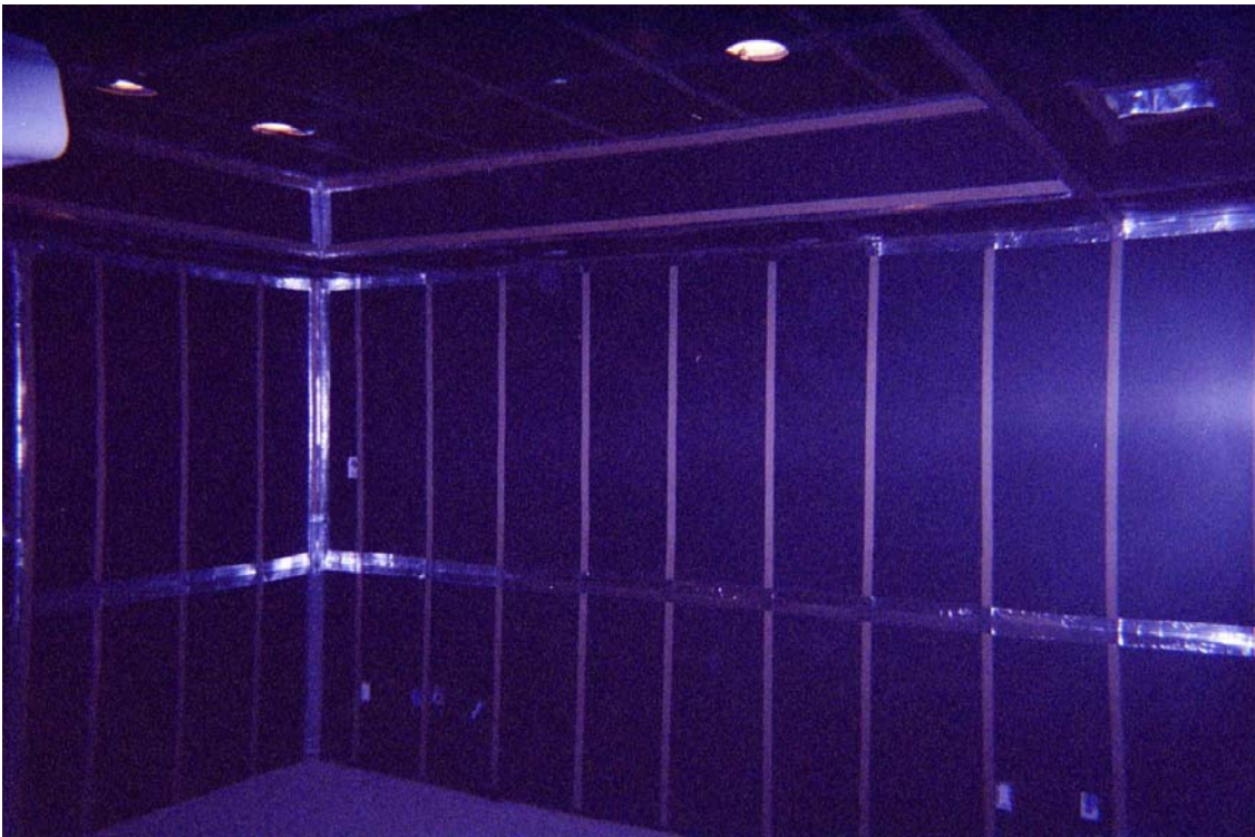
Photo 2 – Finished (rear) wall shown in Photo 1. The foil tape on the flat seams are 4” wide, two 2” applications over the edges of 2” 20 mil PVC tape.
